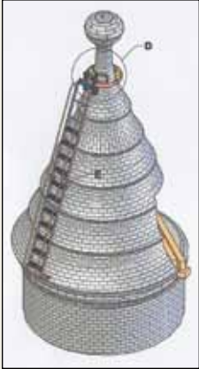
Old Post Office Pavilion , 1100 Pennsylvania Ave., NW, Washington, DC, Phase III. General Contractor: Kaleo Construction, LLC. Replace slate and flashings on 17 dormers and restore masonry. Unique ladder design used to restore the masonry on 8 towers saves GSA money for scaffolding.
