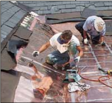
National Presbyterian Church , 4101 Nebraska Avenue, NW, Washington, DC, Phase II. NPC Project Managers: Tony LeManger and Larry Eighmy, Stonehouse Group. New flat seam copper roofs.
