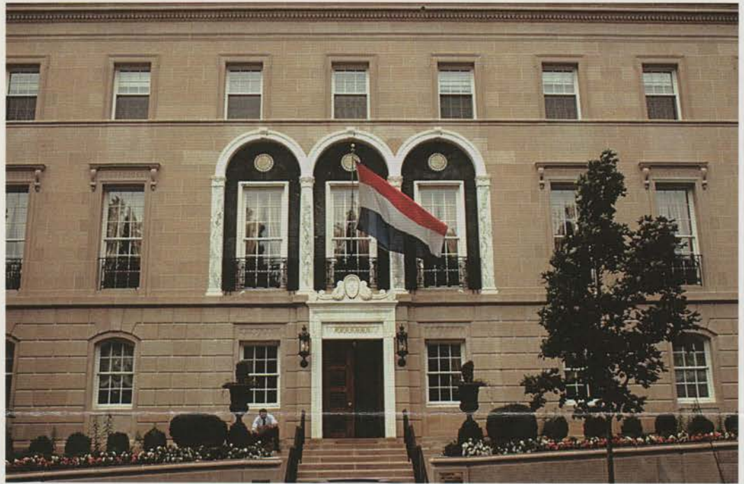
This neoclassical-revival mansion owned by the Netherlands is both the ambassador's home and a private museum. Renovating the mansion's exterior and interior was a complex five-year international project. Wagner replaced all roofing above the gutter line.
